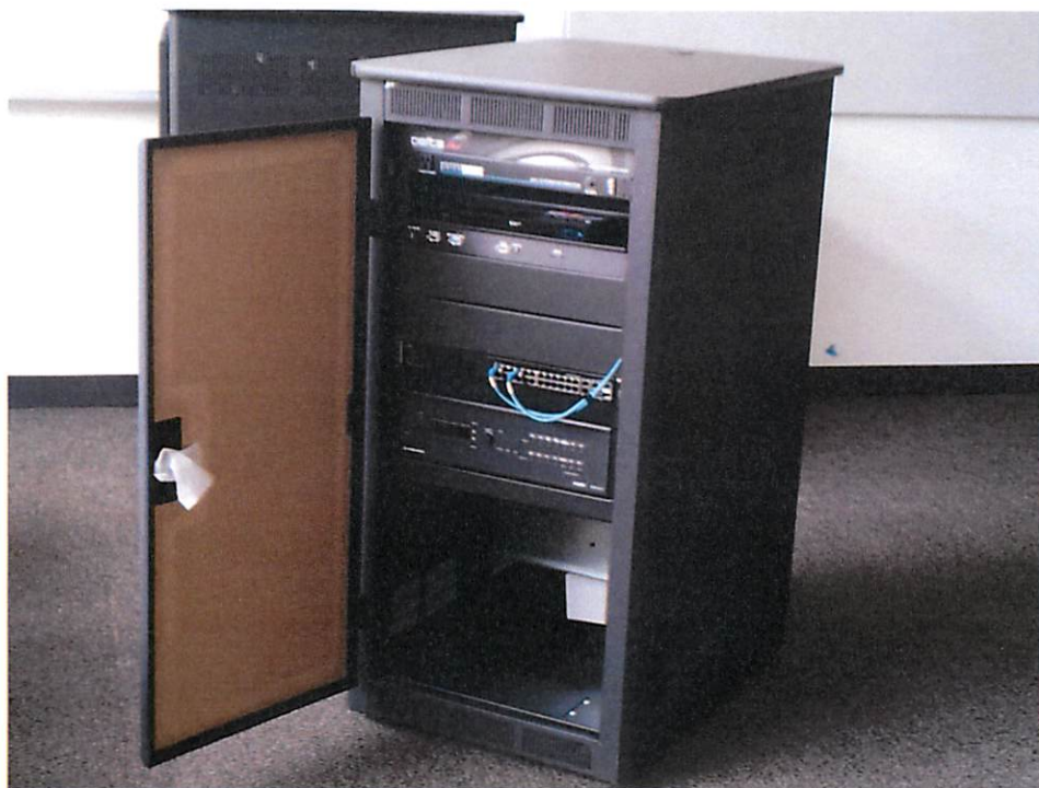
Conference Room Video Routing Equipment – Health Careers, 150
