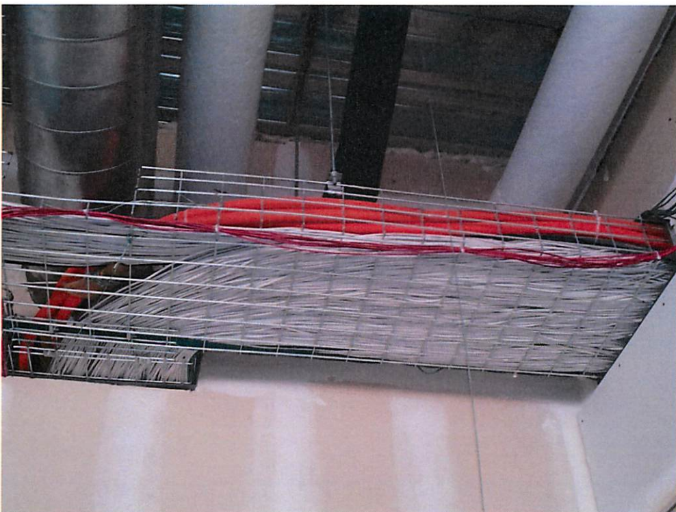
Over 1,000 data cables exiting the data closet – Science Building, Cable Tray
