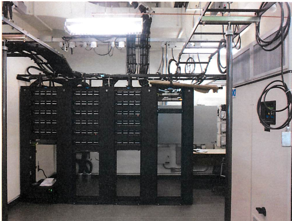
Completion of Data Rack Installation – Health Careers, MDF
