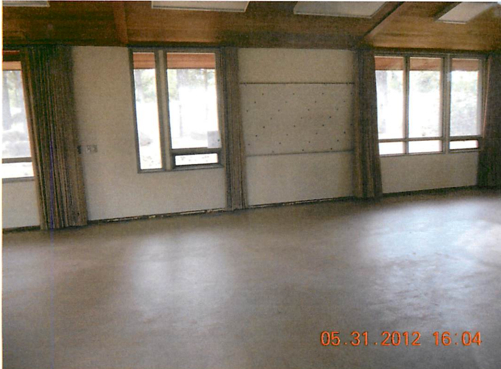
Upper meeting room complete with exception of rubber base and bathroom door trim.
