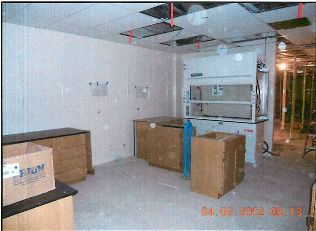
First floor prep area. Fume hood
