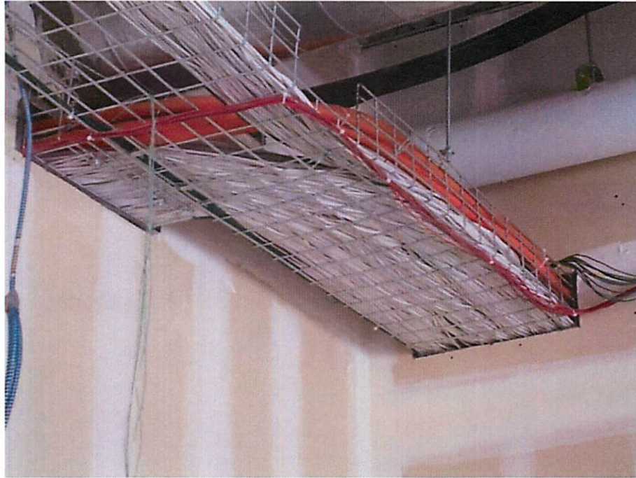
Cable Entry Point to MDF – Science Building, Exterior of MDF, West Wall
