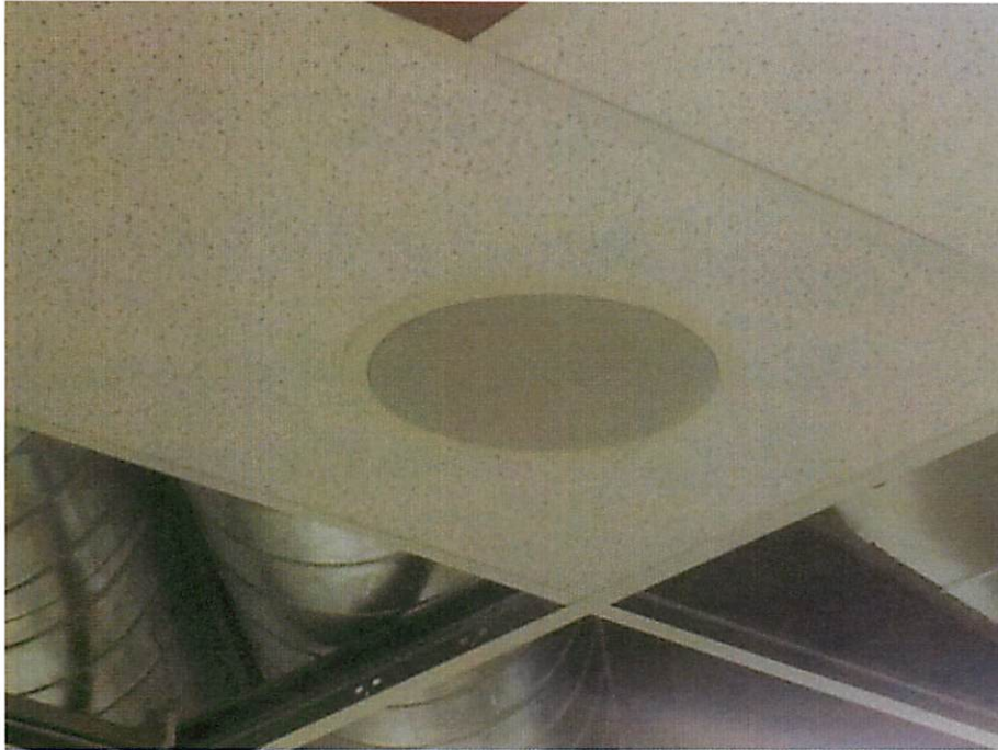
Typical Ceiling Speaker Installation – Science Building, First Floor
