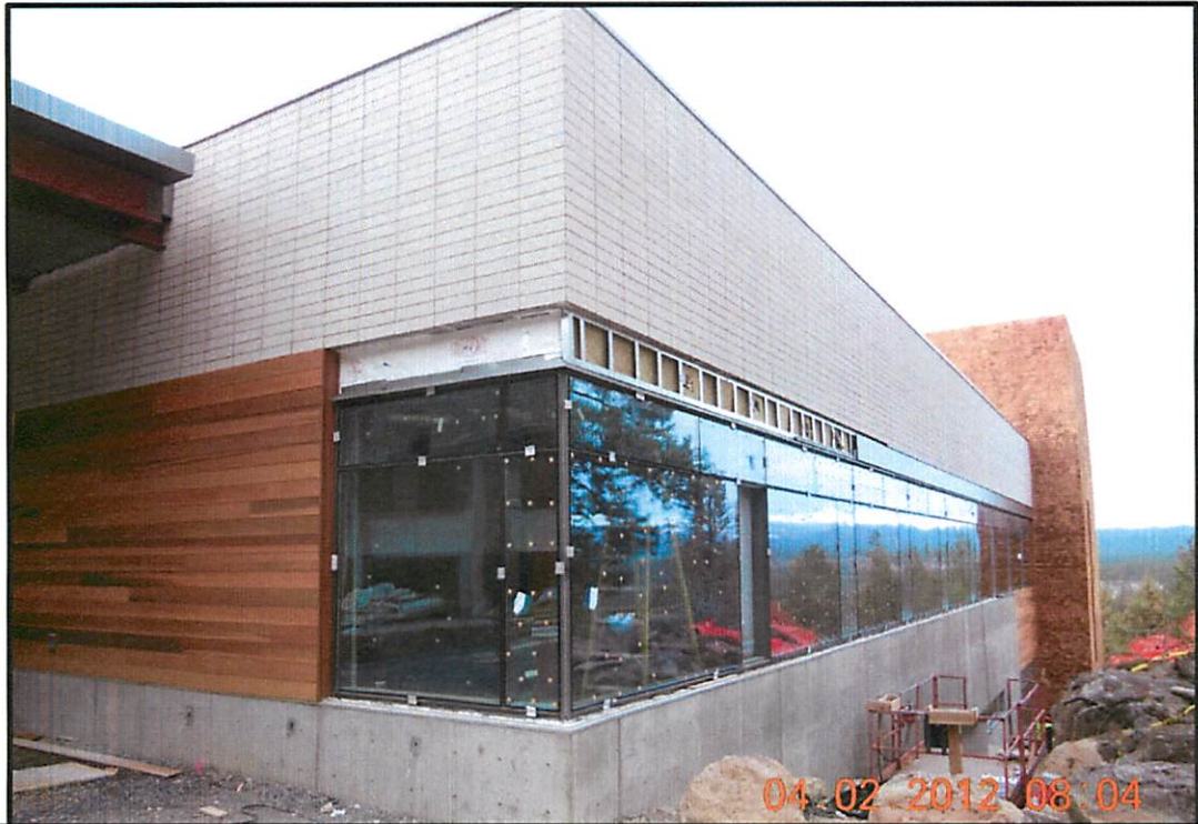
North Elevation: Wood shingle and lap siding work complete. Window system in place and metal panel progressing.
