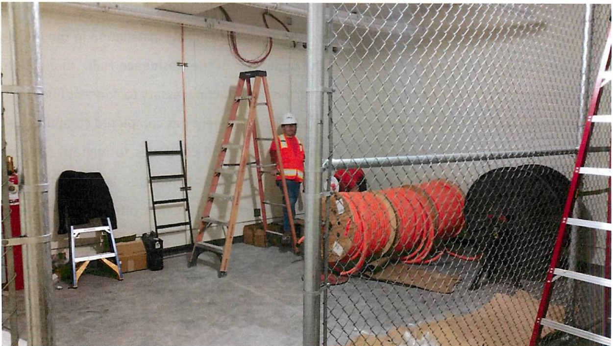
Network Innerduct and Coaxial Cable Installation - MDF
