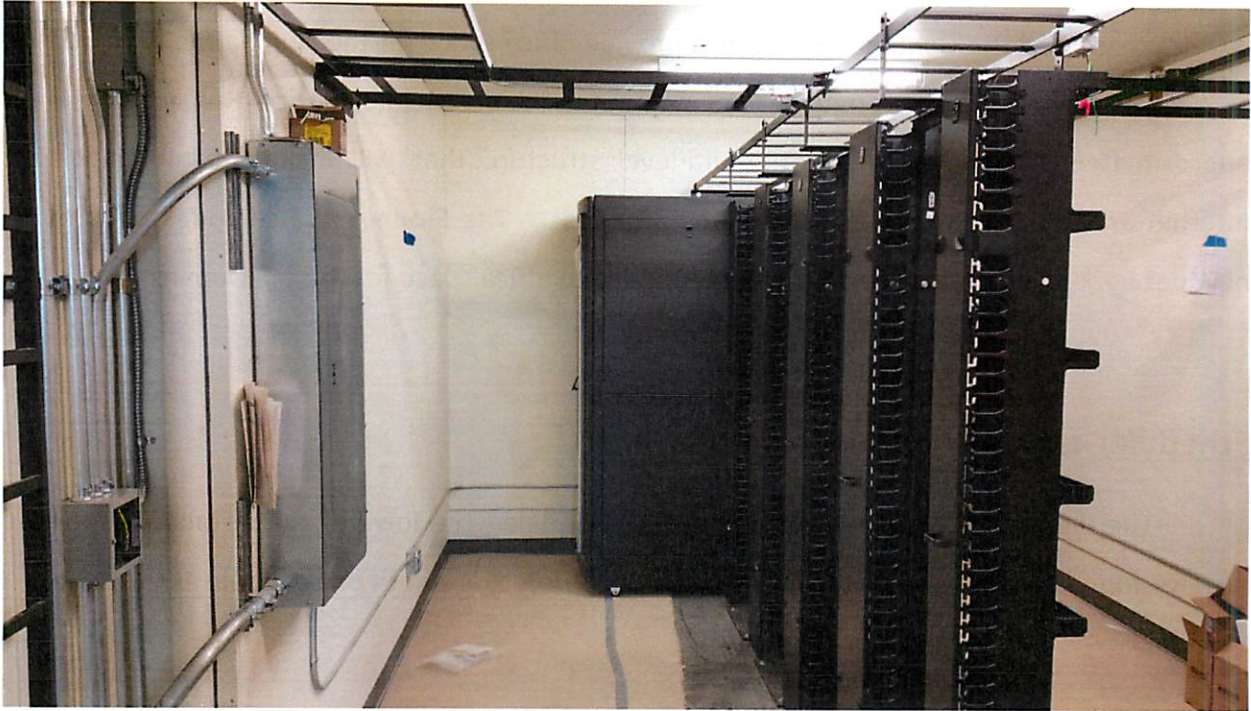
Telephone and Fiber rack installation - IDF
