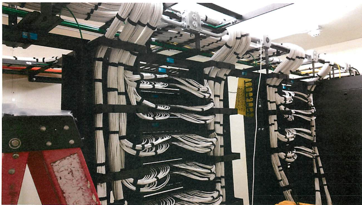
Network Cable Installation – Residence Hall, IDF
