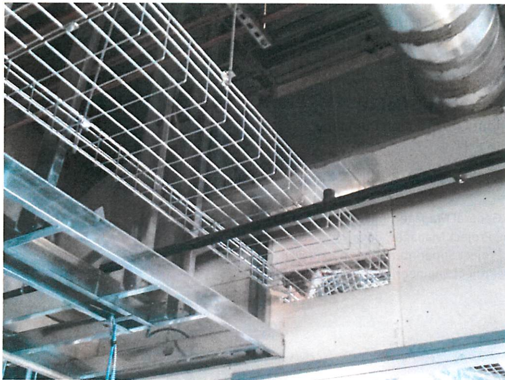
Data & AV Cable Tray – Science Building, First Floor
