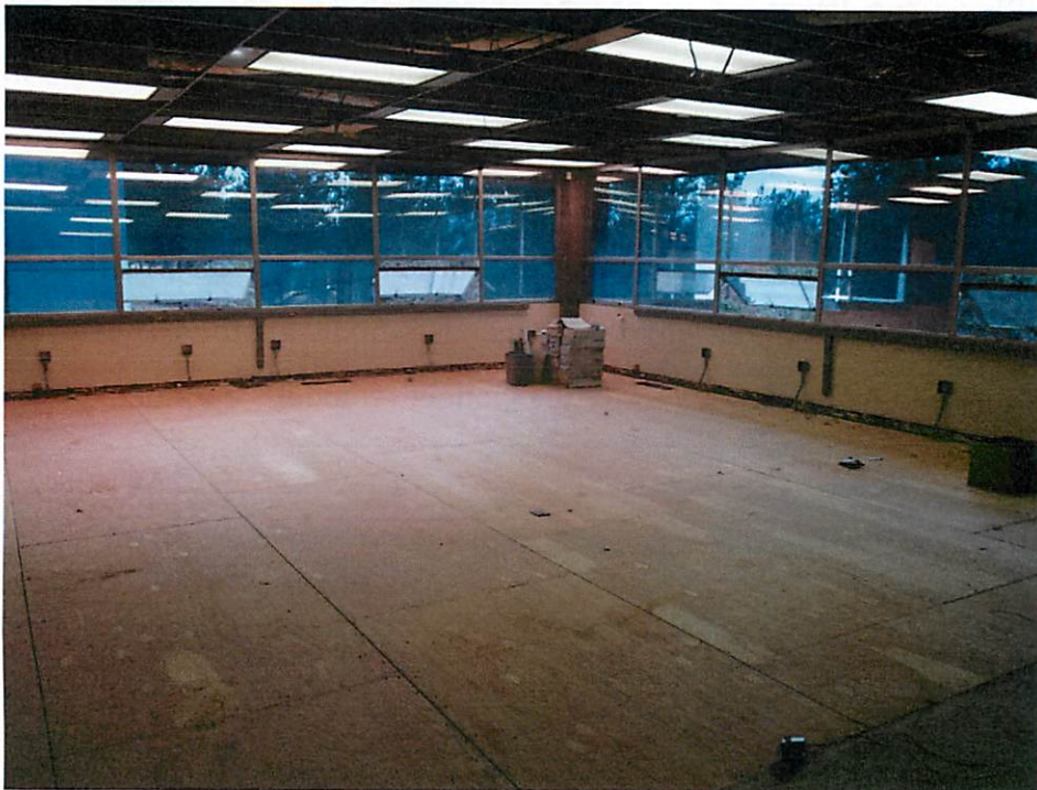
Low-voltage Floorbox and Wall Outlets – Pioneer 232
