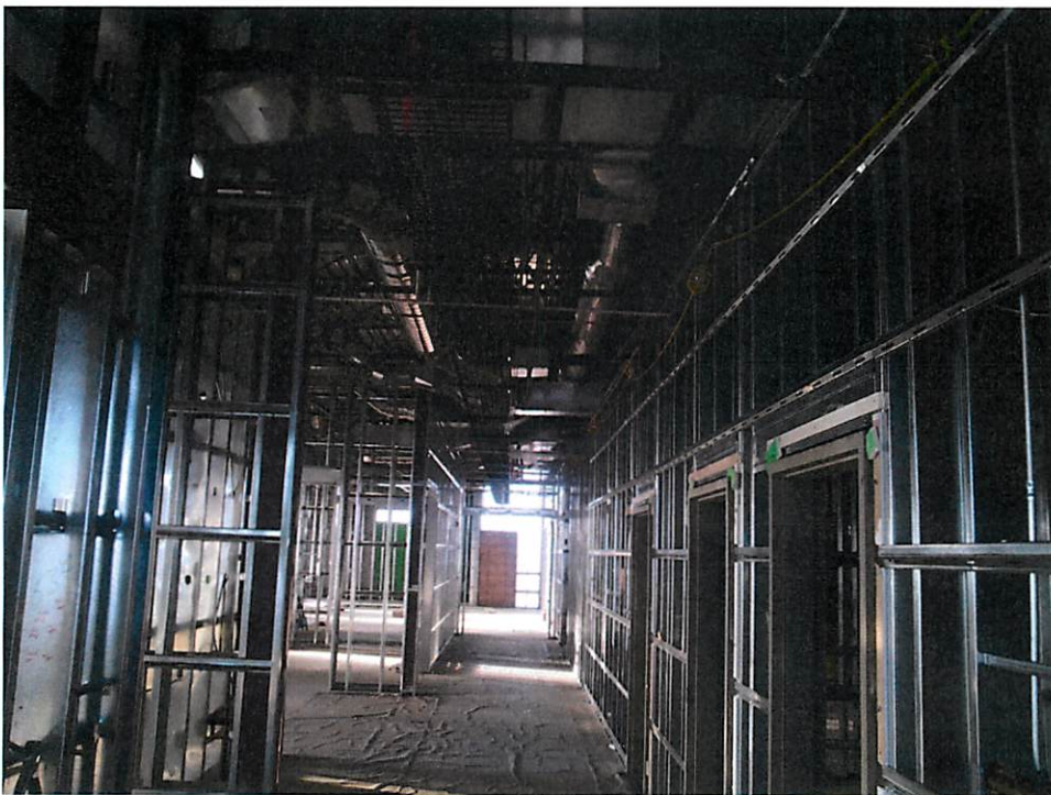
Low-Voltage Cable Tray – South Wing, 2 nd floor
