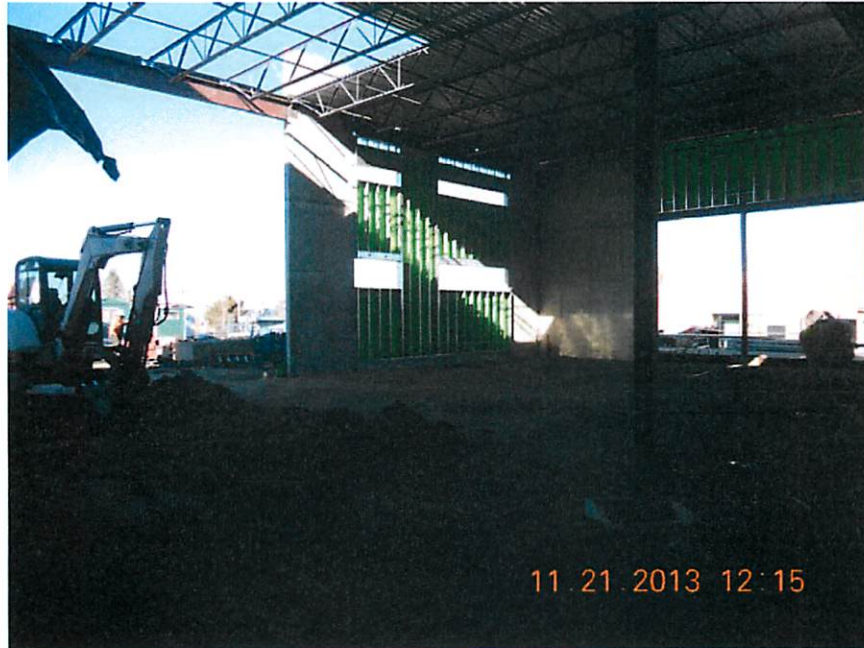
North Wing – NDT/NDI Area
