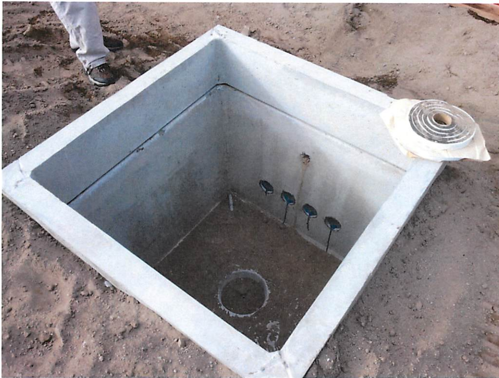
Data & Telecom Vault – Redmond Building One
